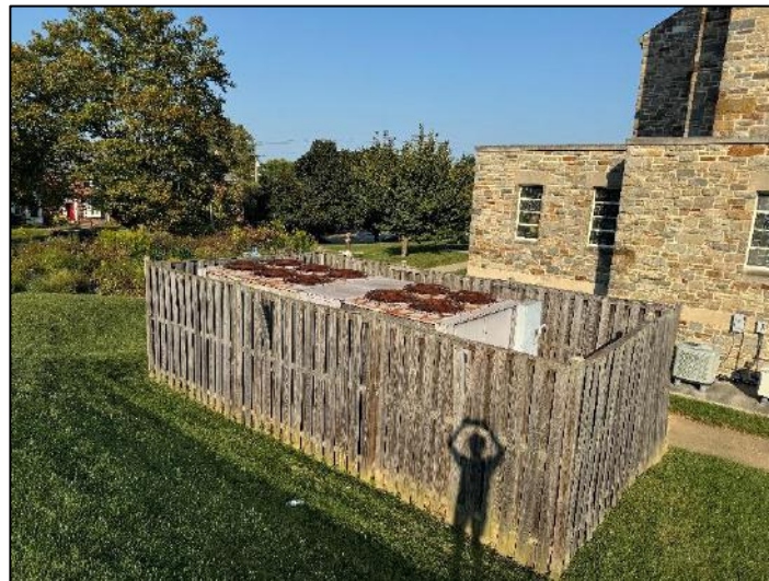
Photo 4b: Existing Chilled Water System
