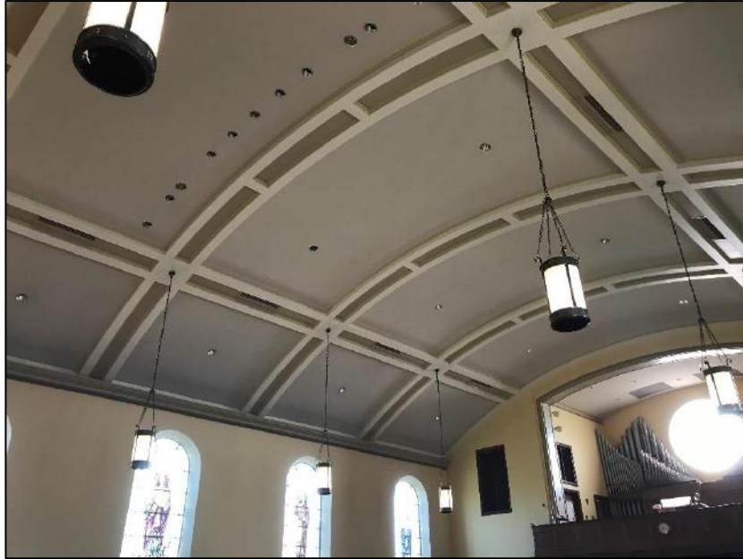
Photo 7: Interior Lighting Systems
