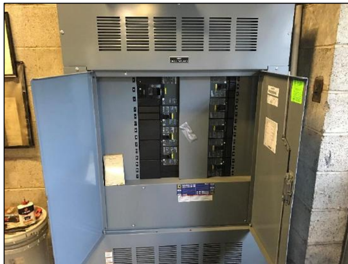
Photo 6: Existing Electrical System
